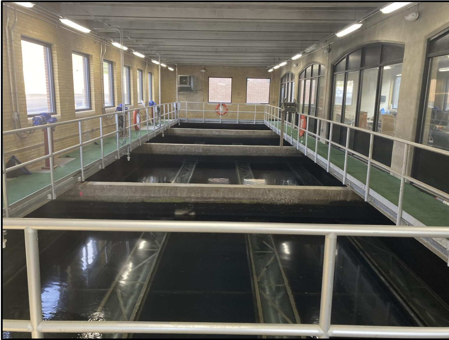
Dual Media Filters (Sand and Anthracite) at Observatory Water Treatment Plant
